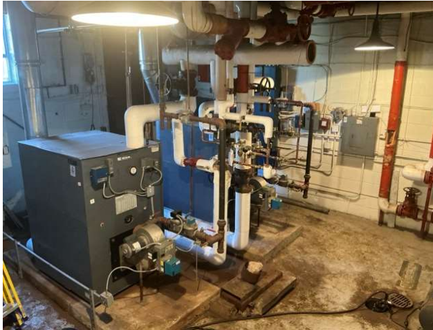
25 - PRESCHOOL BOILERS & PUMPS
