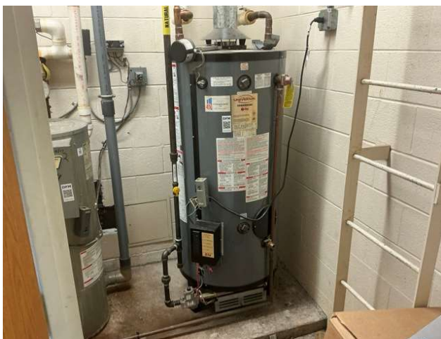
23 - DAYCARE WATER HEATER
