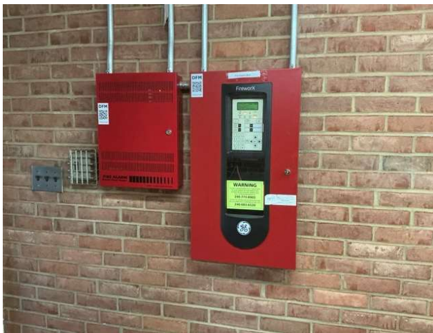
21 - FIRE ALARM PANEL
