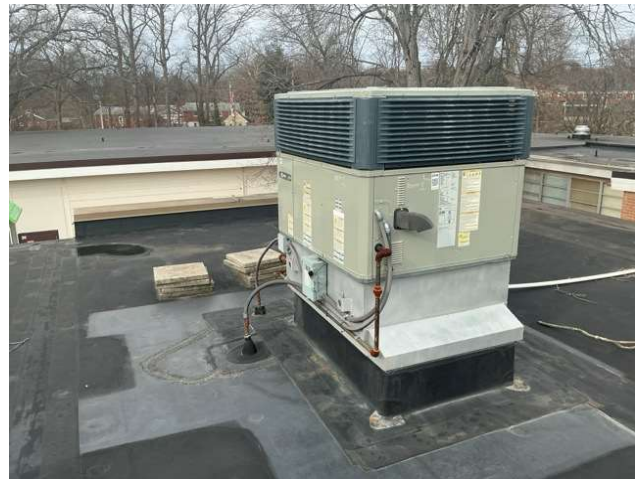
28 - ROOFTOP MECHANICAL EQUIPMENT
